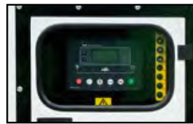
18 CONTROL PANEL PROTECTED FROM RAIN, damage and unwanted access by a locked door.
